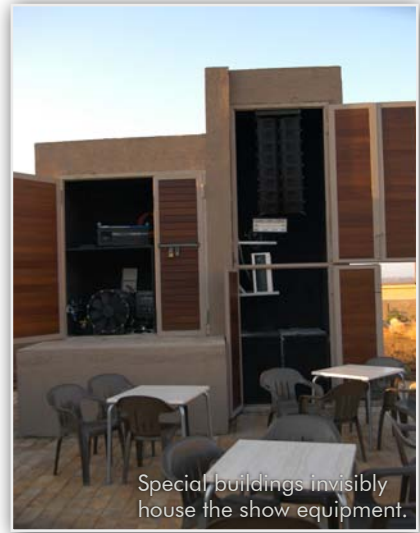
Every evening the park stages a spectacular show, completely automated by a LACON-5 control system.
